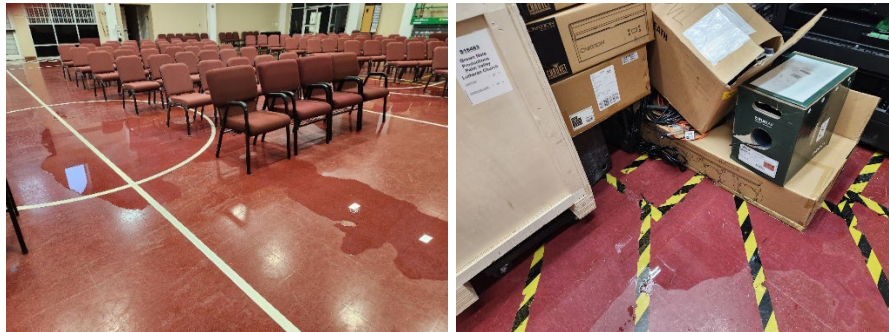
Water issues after heavy rains in June
