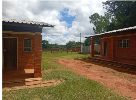
We have come along the students' block and are at the top of that block. On the right hand side are the first of the storerooms.
