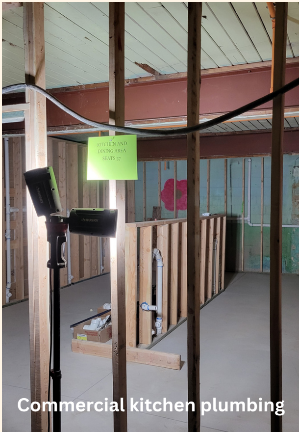
Transformational Housing HVAC ducting & plumbing
